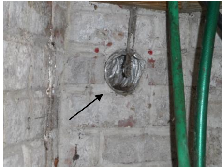
Missing vent cover for vent under deck.
