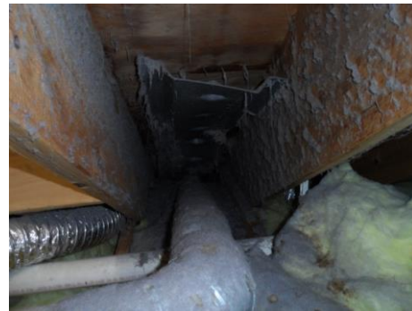
Dry vent backing up into attic.
