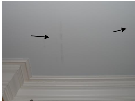
Moisture stains on ceiling in living room.
